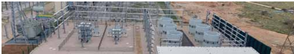
Fig. 18. SVC 250 Mvar in the TS 400/220/110/10 kV Konjsko located near Split Sl. 18. 250 Mvar SVC u TS 400/220/110/10 kV Konjsko blizu Splita
