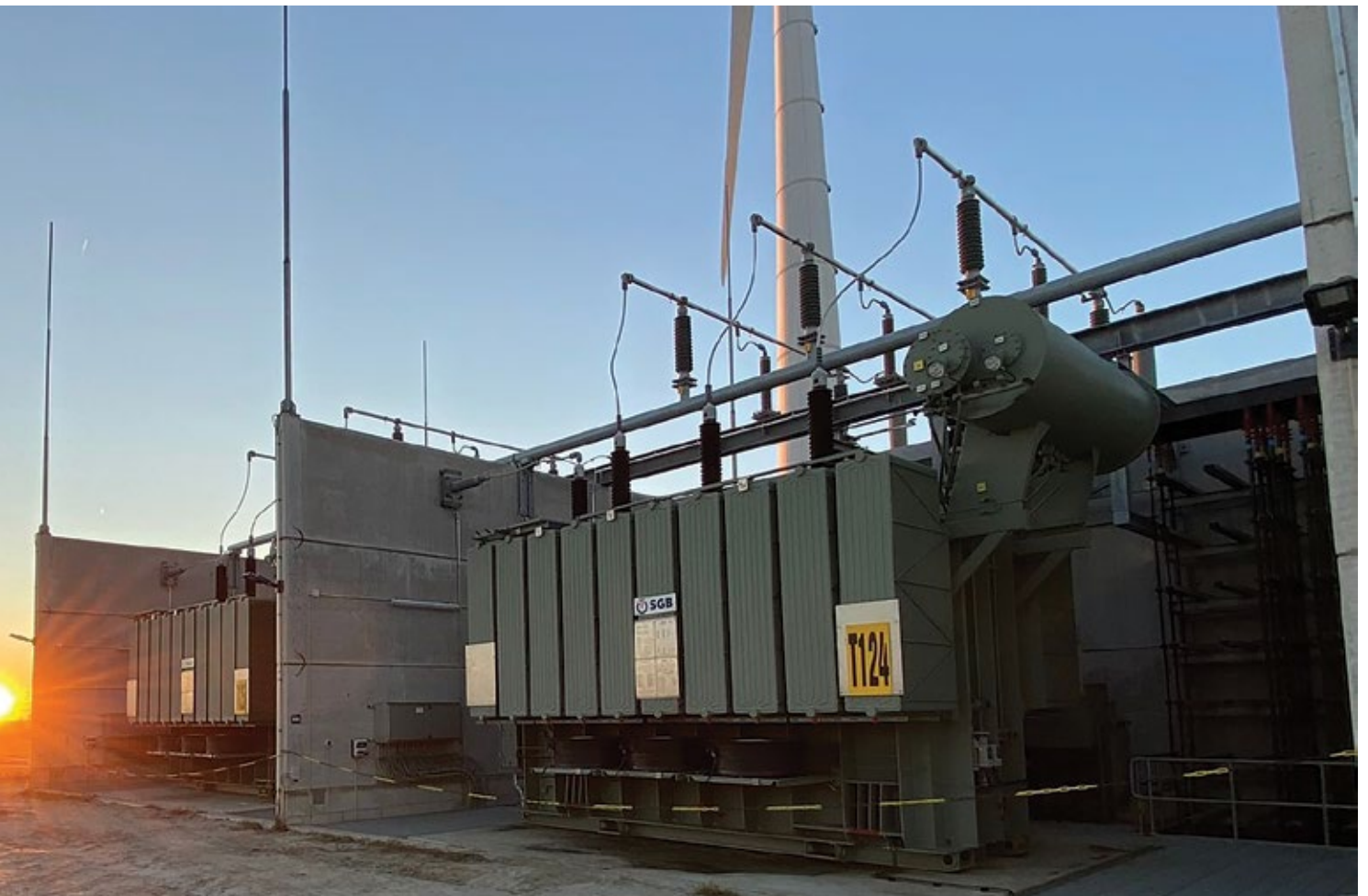
Figure 3. Wind farm substation transformers (photo courtesy of SGB-SMIT)
