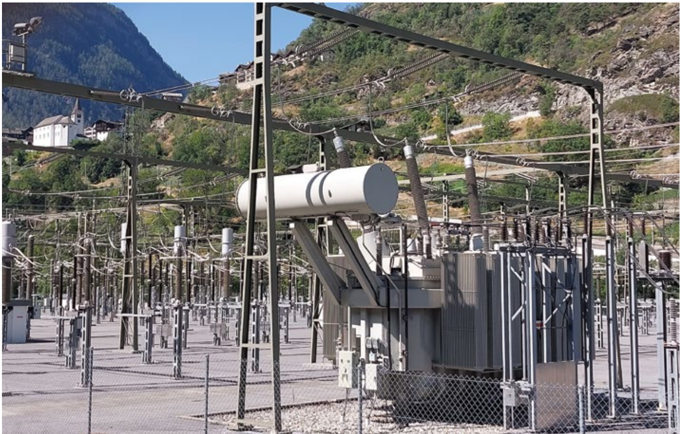
Figure 2. Transformer at the Mattmark hydropower station Stalden in Switzerland
