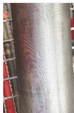
(a) before erosion
