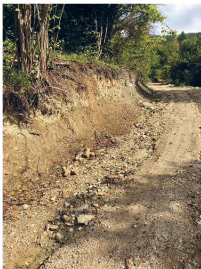
Slika 6. Erozija na kolniku ceste Figure 6. Erosion on road pavement
