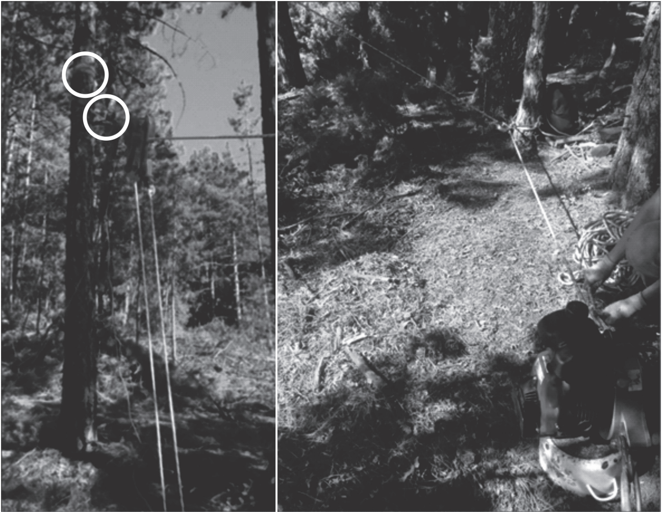
Fig. 4 Installation of skyline (using synthetic ropes and locking device) (left) and portable winch (right) at landing area
