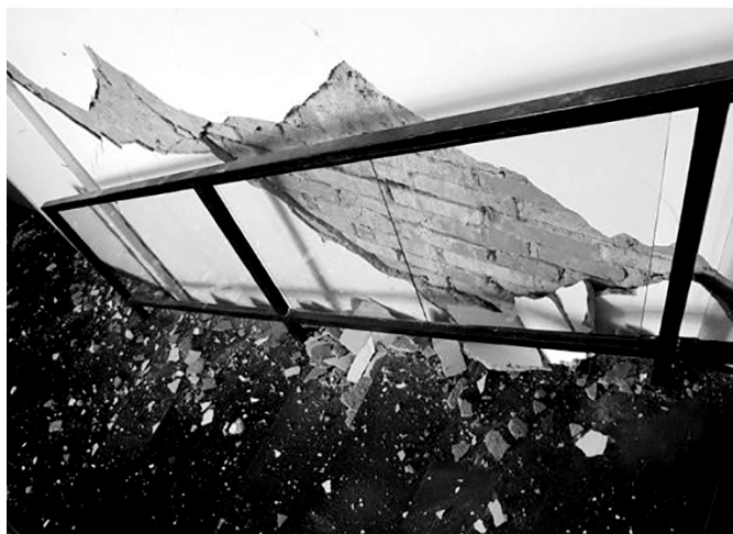
Figure 1. Damaged walls of the Institute of Art History after the earthquake of March 22, 2020. (Photo: Danko Zelić)
