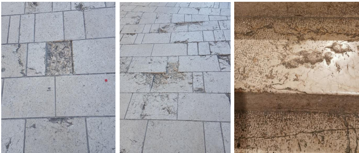
Figures 10-12: Non-uniformity of cracks and damage in the busy pedestrian zone of the old town of Sarajevo (left and middle), as well as the original internal stairs in the space of the BiH Art Gallery in Sarajevo 10
