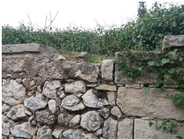
Figure 8. Absence of concrete cap
