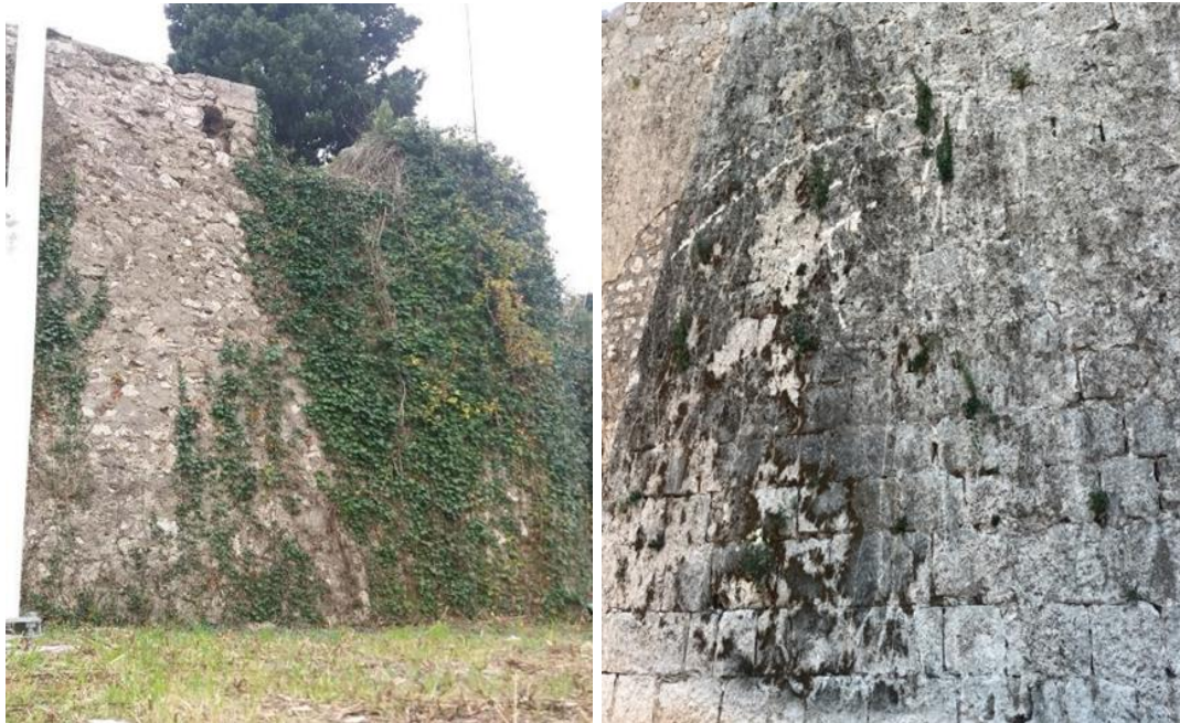
Figure 5. The outer surface of the wall covered with vegetation and its condition after its removal
