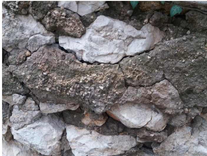
Figure 7. Separation of mortar
