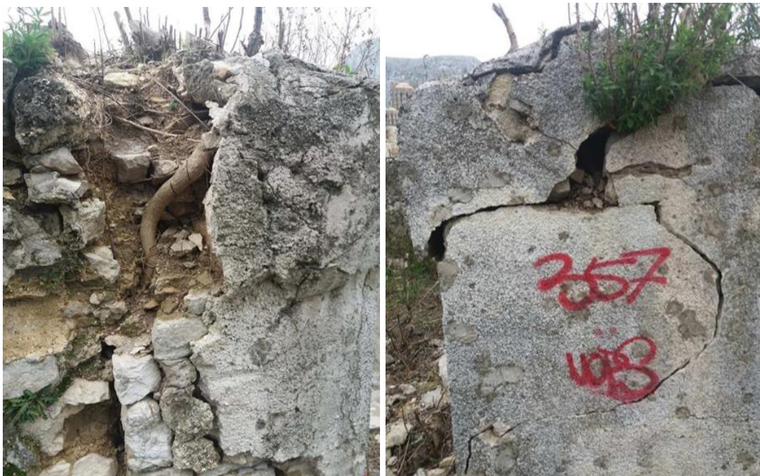
Figure 6. Damage caused by root action
