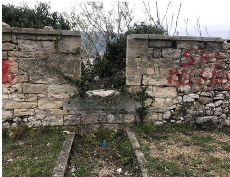
Figure 10. Graffiti on the structure
