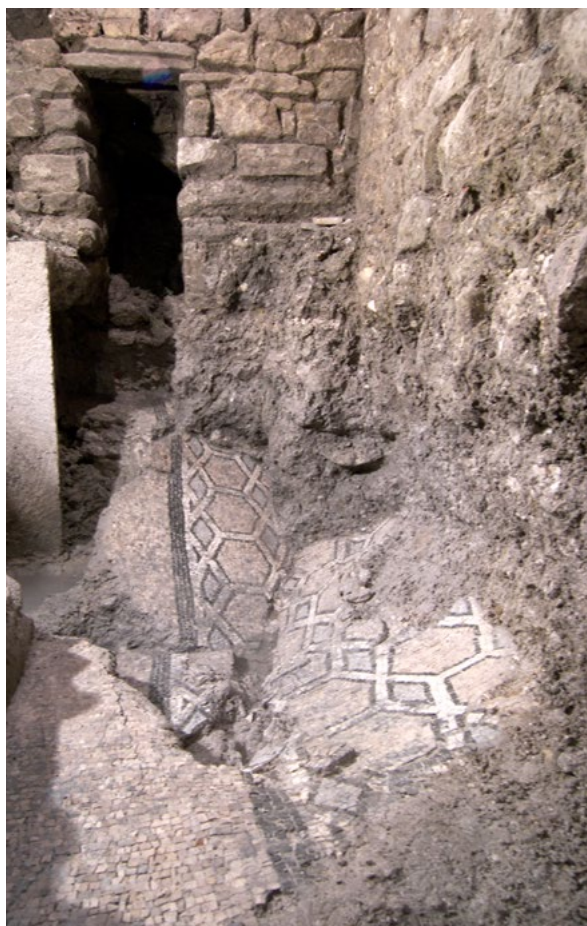
8. Dio mozaika u Arhiđakonovoj 1 oštećen zidom srednjovjekovne kuće i protokom vode (fototeka KO-ST, snimka: V. Kovačić, 2010.) Part of the mosaic in Arhiđakonova 1 damaged by the wall of a medieval house and the flow of water (KO-ST Photo Archive, V. Kovačić, 2010)
