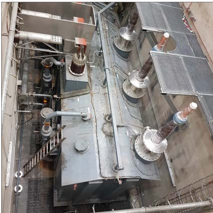
Figure 5. 400 kV / 250 MVA monitored transformer
