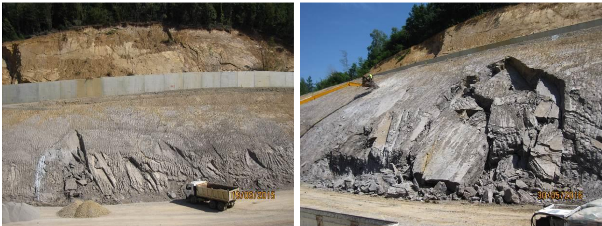
Figure 3. and 4. Planar sliding of rock blocks in the highway area
