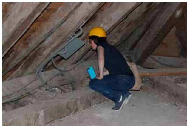
9 Petrinja, zgrada Suda, Trg Franje Tuđmana 12, Katrin Beyer s Federalnog tehnološkog instituta u Lausanni (EPFL), članica međunarodnog Stručno-savjetodavnog povjerenstva (foto: T. Petrincec, MKM, 2021.) Petrinja, Court building, 12 Franjo Tuđman Square, Katrin Beyer from the University of Lausanne, member of the Expert-Advisory Committee (photo: T. Petrincec, Ministry of Culture and Media, 2021)
