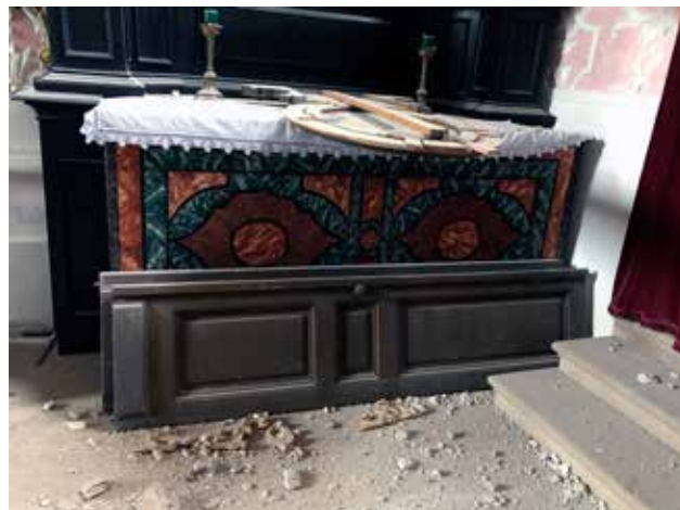
7 Crkva sv. Katarine u Zagrebu, oštećenje slike sv. Arkandela Rafaela s oltara sv. Barbare uslijed pada s atike (foto: Z. Mažar, GZZSKP 2020.) Church of St. Catherine in Zagreb, damage to the retable of St. Archangel Raphael from the altar of St. Barbara as a result of its collapse from the attic (photo: Z. Mažar, City Institute for the Conservation of Cultural and Natural Heritage, 2020)
