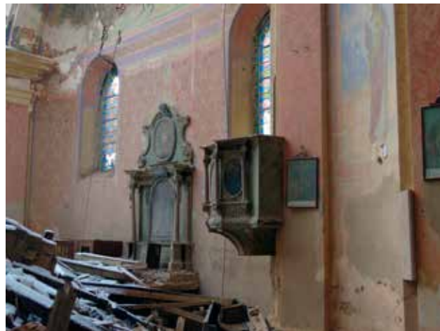
6 Crkva sv. Nikole i Vida u Žazini, bočni oltar Majke Božje Žalosne oštećen uslijed urušavanja svoda (foto: T. Horvatić, MKM, 2021.) Church of St. Nicholas and Vitus in Žazina, the lateral altar of Our Lady of Sorrows damaged due to the vault's collapse (photo: T. Horvatić, Ministry of Culture and Media, 2021)
