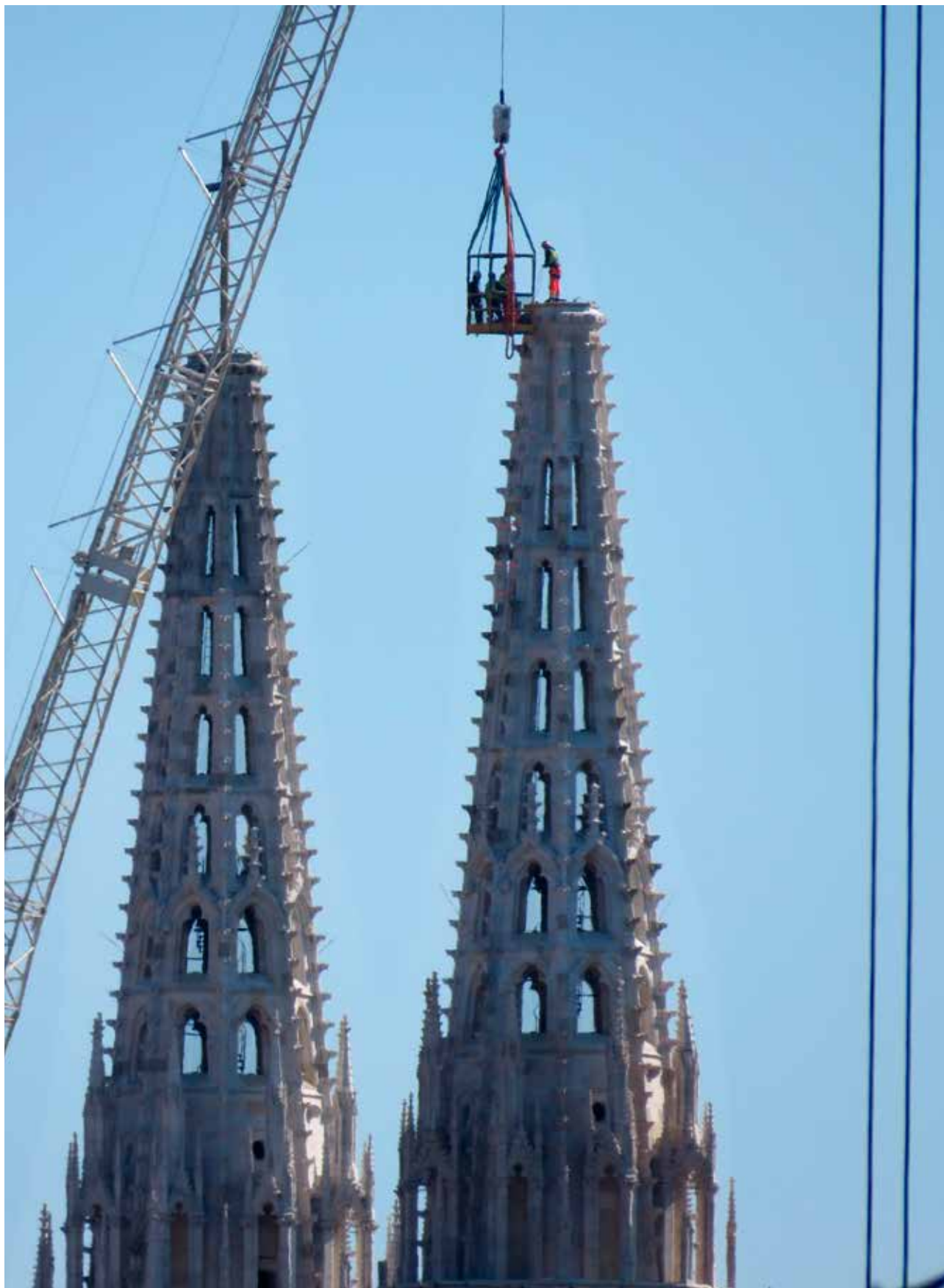
Heavy damage to the bell towers of the Cathedral of the Assumption of the Blessed Virgin Mary and St. Stephen and St. Ladislaus in Zagreb after the 2020 earthquakes (photo: G. Jerabek, Ministry of Culture and Meida, 2021)
