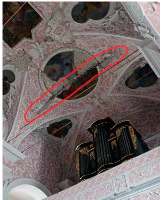
12 Possible constructive joint running along the upper choir arch (photo: X. Romão, July 2021)
