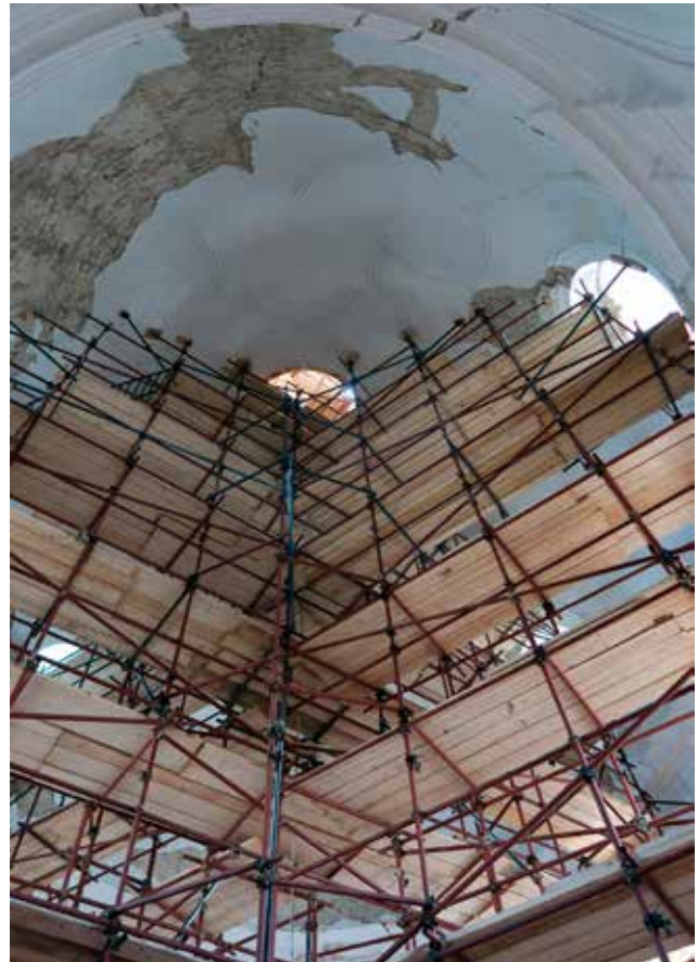
20 Vault shoring in the central zone of the dome showing missing parts of the finishings (photo: X. Romão, July 2021)
