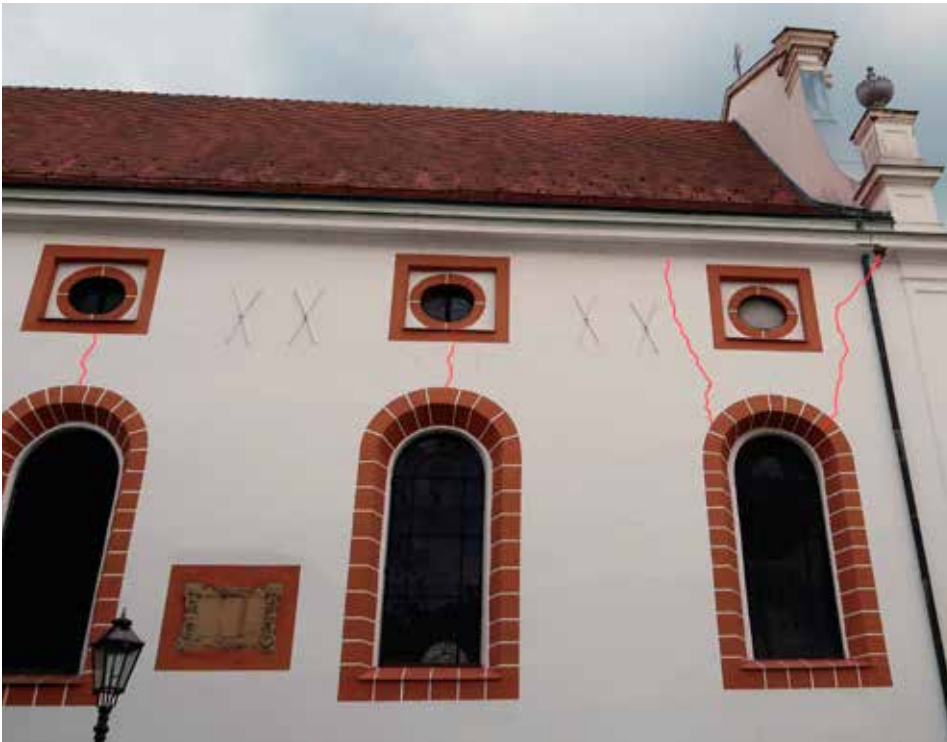
6 General view of the external damage of the church, where there is no evidence of masonry crushing at the anchorage zones of the tie rods (photo: X. Romão, July 2021)
