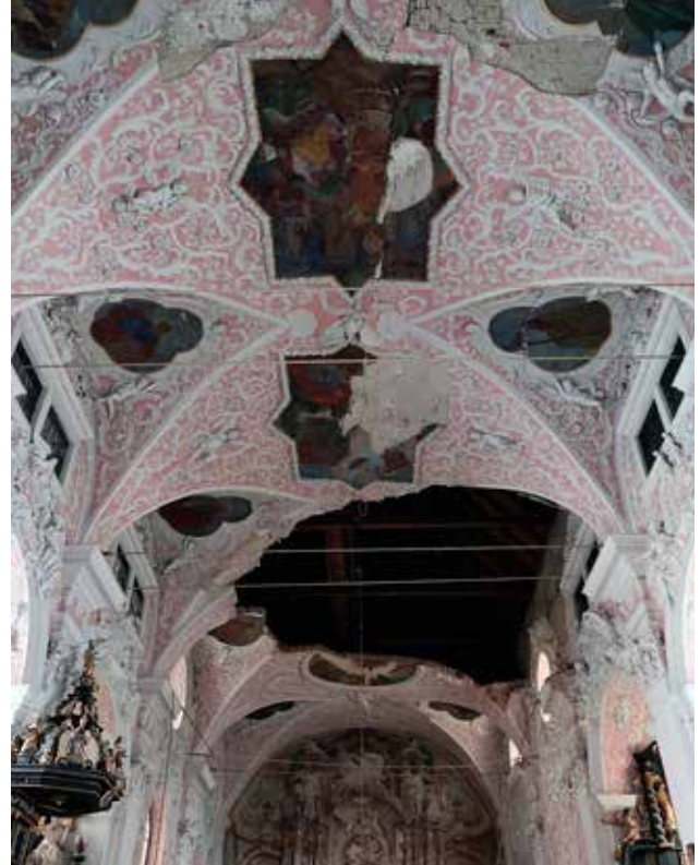
10 Longitudinal cracking along the vault crown line (photo: X. Romão, July 2021)
