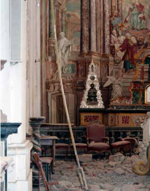
9 Detail of the failure of the triumphal arch tie rod (photo: X. Romão, July 2021)
