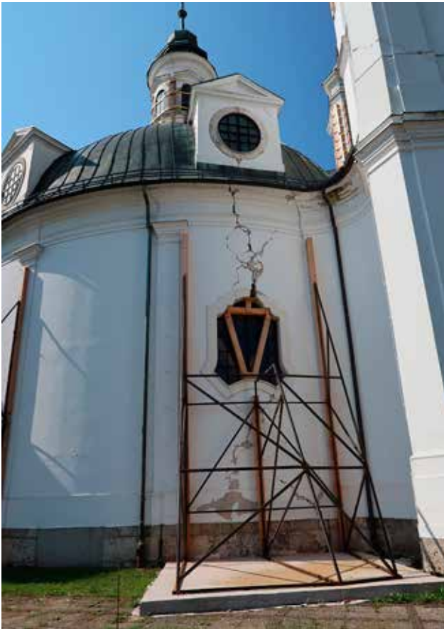
17 External shoring of nave walls in the area of the lateral chapels (photo: X. Romão, July 2021)
