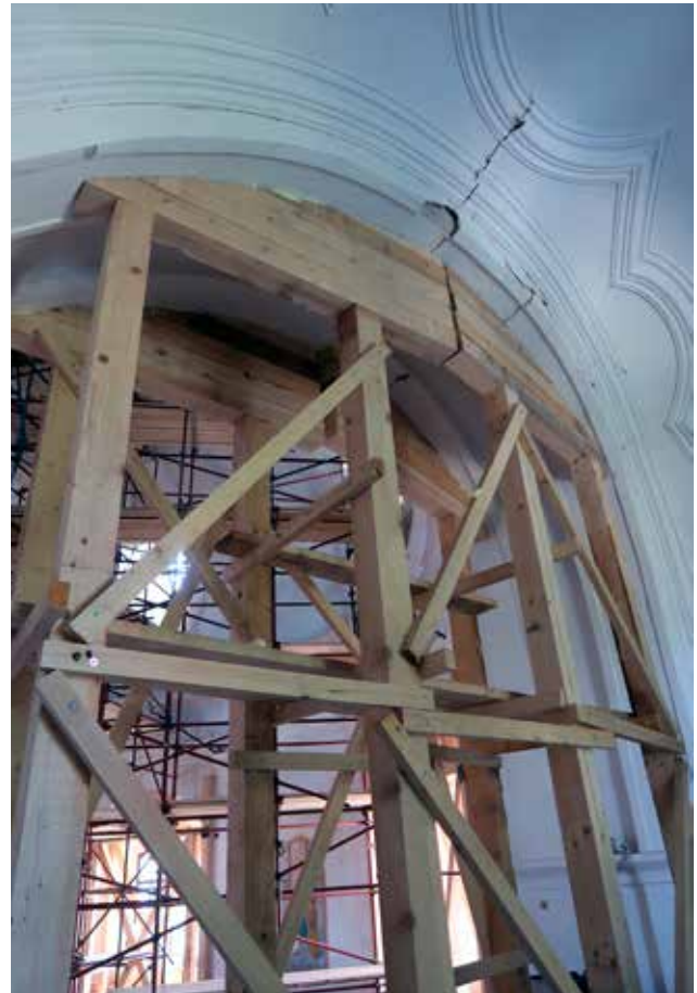
23 Shoring of the arch above the upper-choir which supports the nave vault (photo: X. Romão, July 2021)
