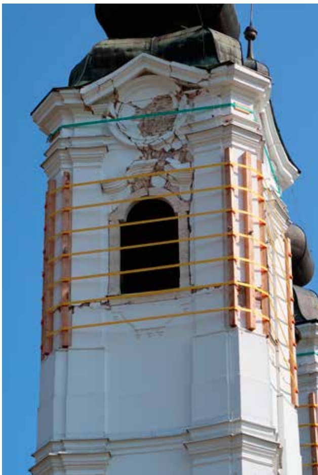
24 Damage in the upper zone of the tower (photo: X. Romão, July 2021)
