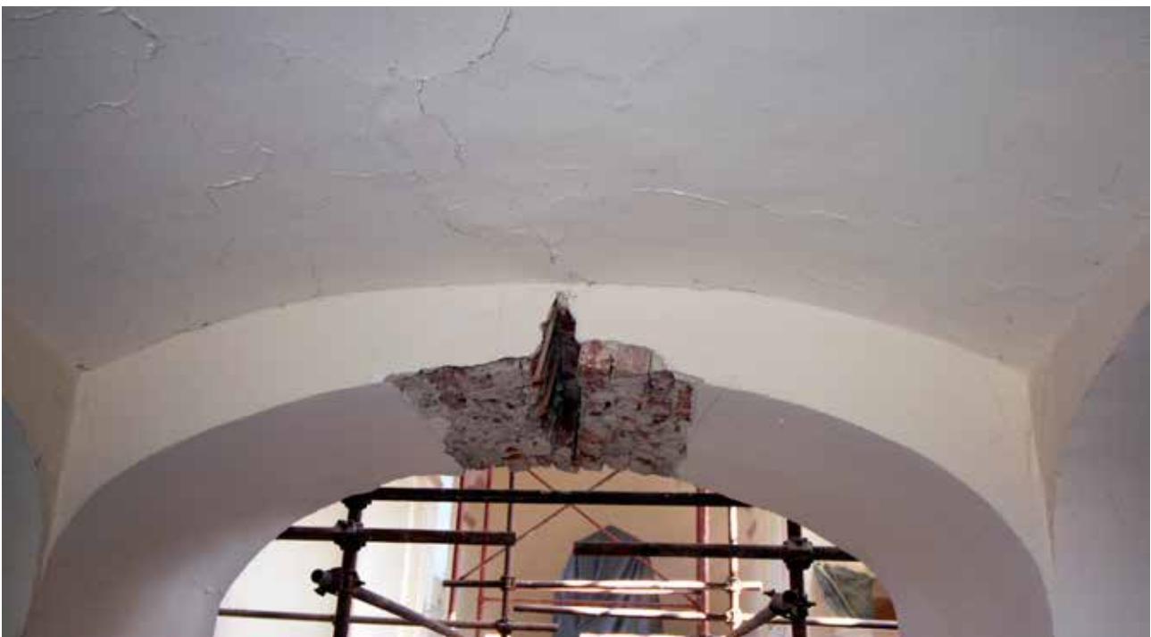
11 Apatovec, crkva sv. Petra, oštećenje lučnog nadvoja kora (foto: M. Pezelj, KO BJ, 2021.) Apatovec, Church of St. Peter, damage to the arched vault of the choir (photo: M. Pezelj, Conservation Department Bjelovar, 2021)
