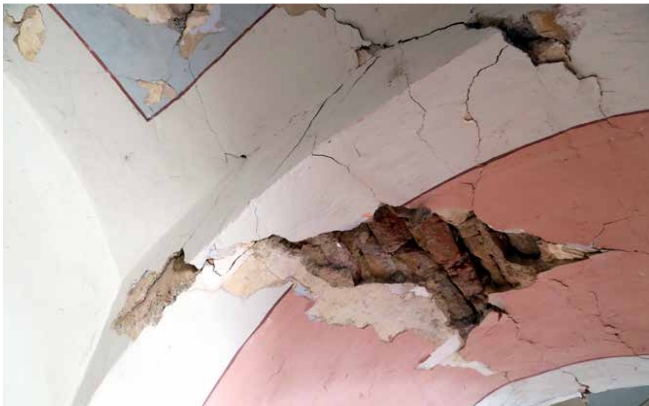
12 Mali Raven, crkva sv. Ladislava i Presvetog Srca Isusova, oštećenje lučnog nadvoja i svoda kora (foto M. Pezelj, KO BJ, 2021.) Mali Raven, Church of St. Ladislau and the Sacred Heart of Jesus, damage to the arched lintel and vault of the choir (photo: M. Pezelj, Conservation Department Bjelovar, 2021)
