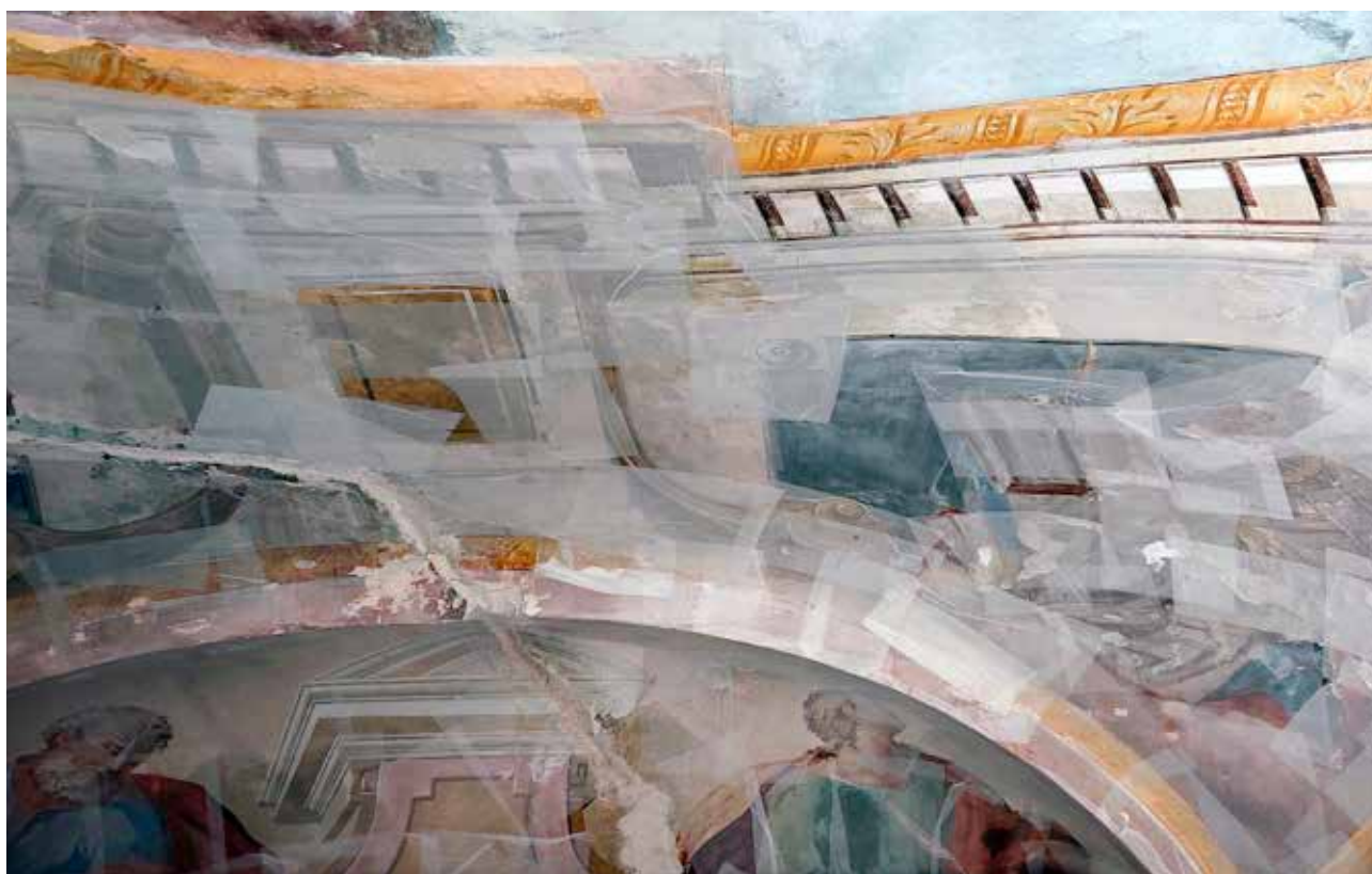
13 Legrad, crkva Presvetog Trojstva, stabilizacija zidnog oslika japan papirom (foto: M. Pezelj, KO BJ, 2022.) Legrad, Church of the Holy Trinity, stabilization of wall painting with Washi paper (photo: M. Pezelj, Conservation Department Bjelovar, 2022)
