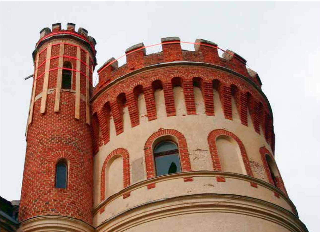
10 Dioš, dvorac Dioš, hitne mjere zaštite stubišnog rizalita i sjeveroistočne kule zatezanjem (foto: M. Pezelj, KO BJ, 2022.) Dioš, Dioš Castle, emergency protection measures of the staircase flights and the northeastern tower by tensioning (photo: M. Pezelj, Conservation Department Bjelovar, 2022)
