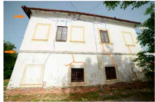
15 Identification of the cracks belonging to in-plane failure modes for the east façade (photo and drawing: Thibaud Maillard, 2023)
