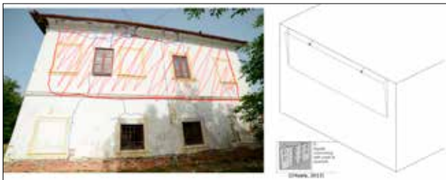
19 Out-of-plane mechanism n°2 in the east façade (photo and drawing: Thibaud Maillard, 2023)
