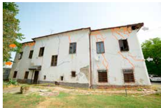
13 Identification of the cracks belonging to in-plane failure modes for the south façade (photo and drawing: Thibaud Maillard, 2023)
