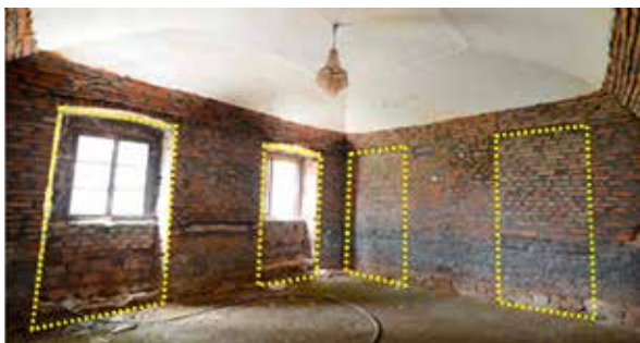
8 Examples of infilled masonry portions considered as openings in the EFM (photo and drawing: Thibaud Maillard, 2023)
