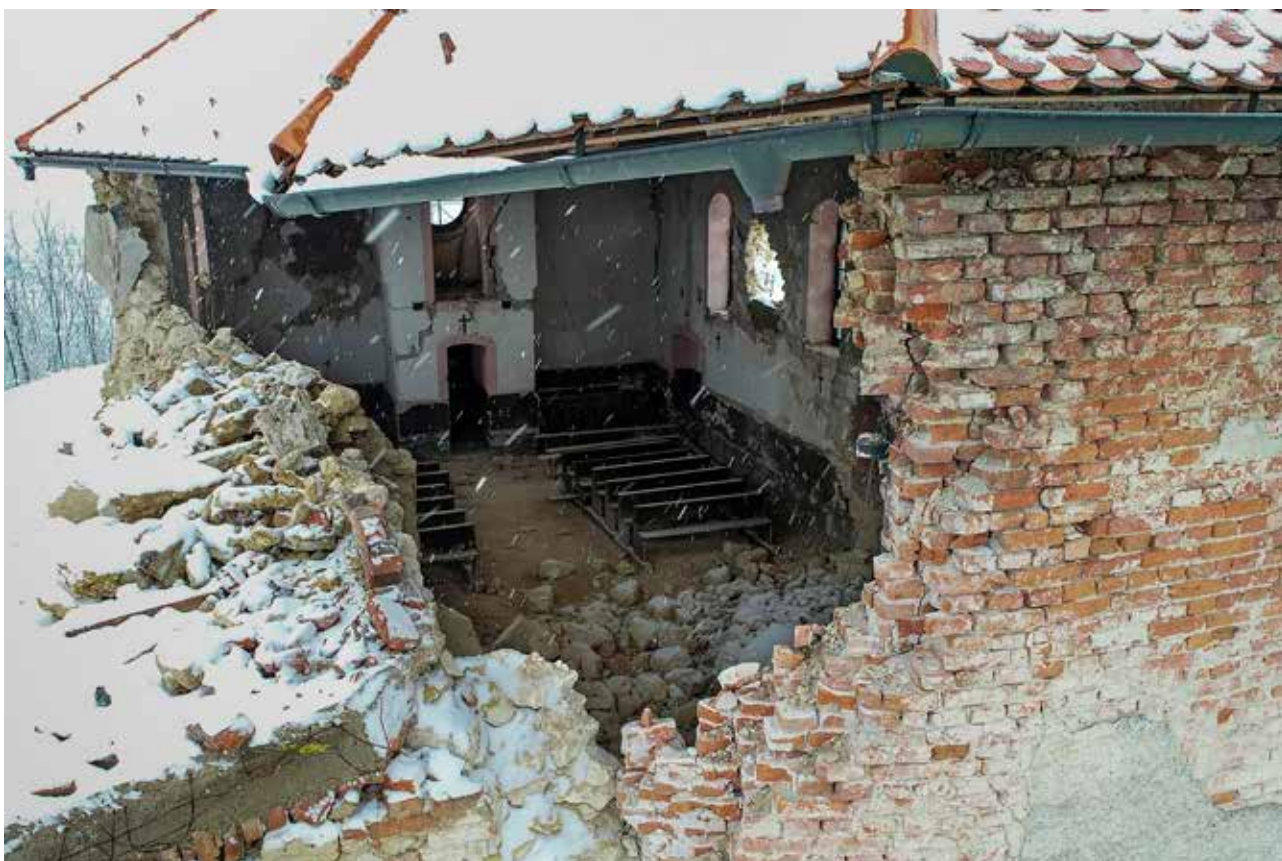
13 Kapela Presvetog Trojstva, oštećenja u potresu, prosinac 2020. (foto: I. Kralj, https://ika.hkm.hr ) Chapel of the Holy Trinity, earthquake damage, December 2020 (photo: I. Kralj, https://ika.hkm.hr )
