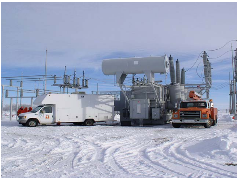
Figure 1. Transformer during test activities
