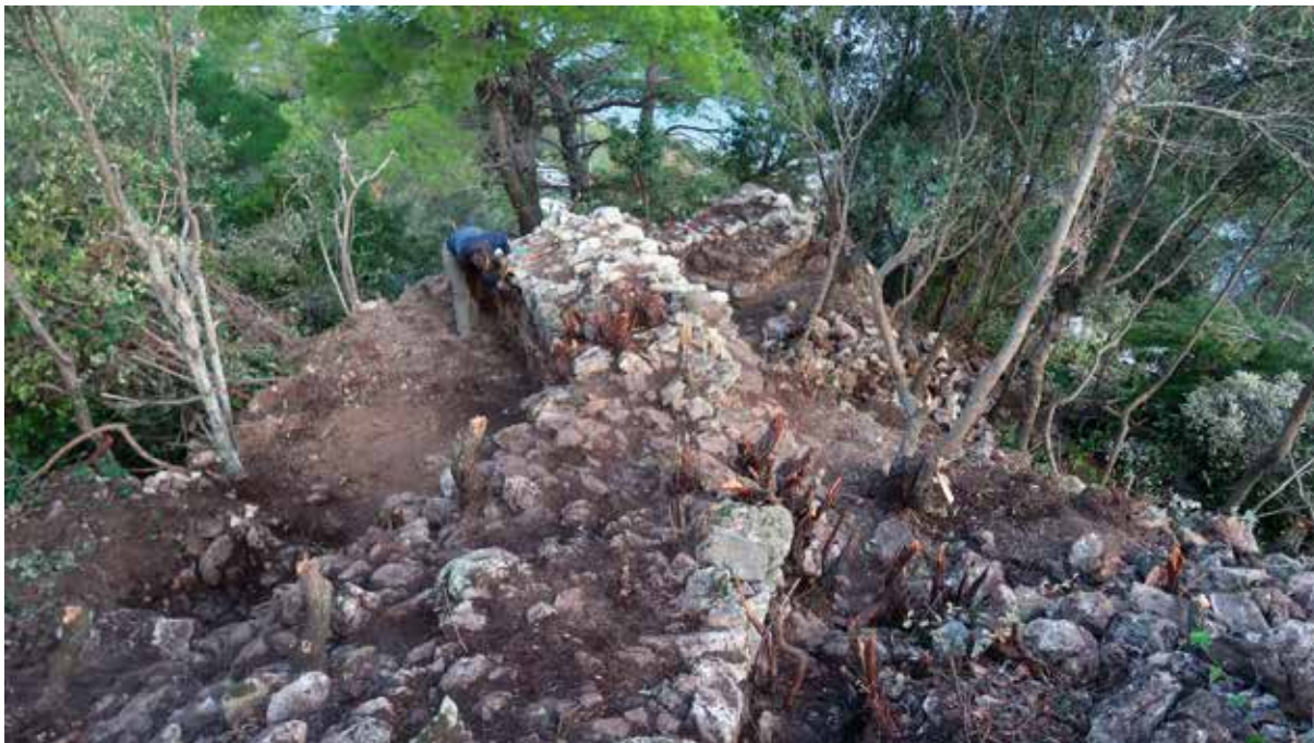
Sl. 6. Pogled s kule na iskopani sjeverozapadni potez bedema Fig. 6 View from the tower onto the north-western stretch of the rampart
