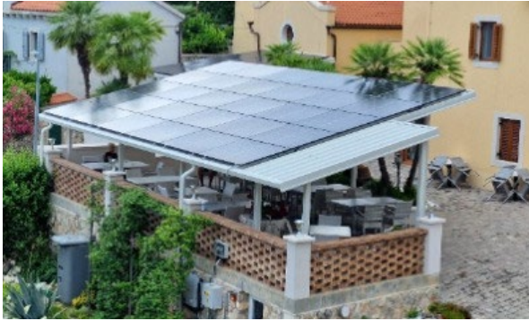
FIGURE 3: PV SYSTEM PHASE SOLAR-2
