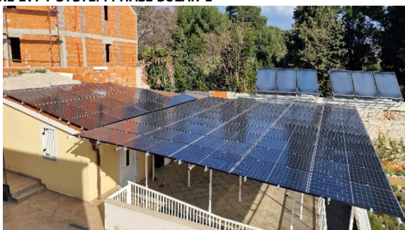
FIGURE 2: PV SYSTEM PHASE SOLAR-1
