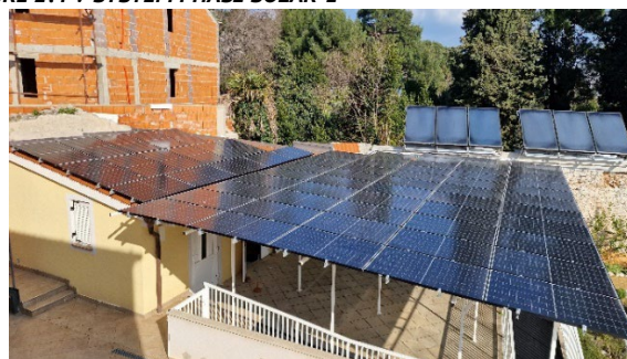
FIGURE 2: PV SYSTEM PHASE SOLAR-1
