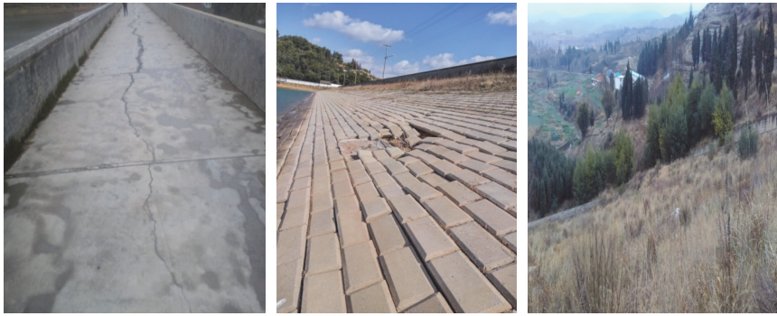
Figure 3. Map of the current condition of the top, face and back of the earth and rock dams
