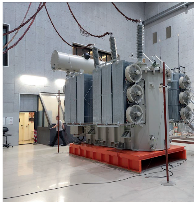
Fig. 6. Power transformer during experiment
