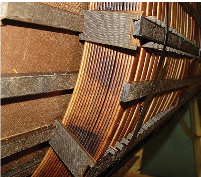
Figure 1. Overheated discs at the top of a winding (ONAF, 66 MVA transformer)
