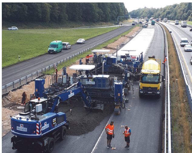
Figure 17. Horizontal-hybrid construction method for the rehabilitation of the heavily traveled A 61 motorway in Germany [7]
