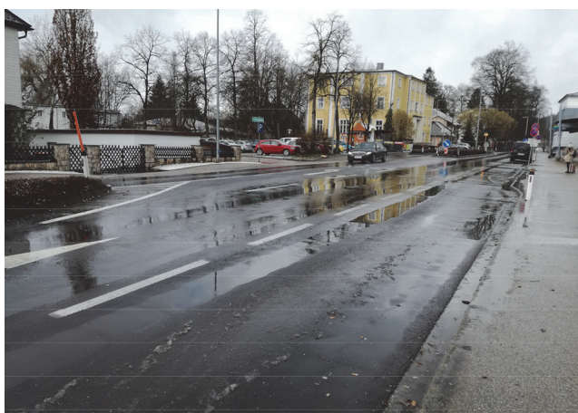
Figure 1. Ruts and deformations in the asphalt by overloading from braking, stopping, and starting at intersections and bus stops [author, 2020]
