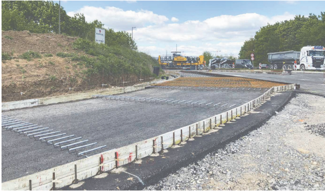
Figure 7. Preparation of concrete layer with reinforced, geometrically critical field; pre-laying of dowels in baskets below the later transverse joint [3]
