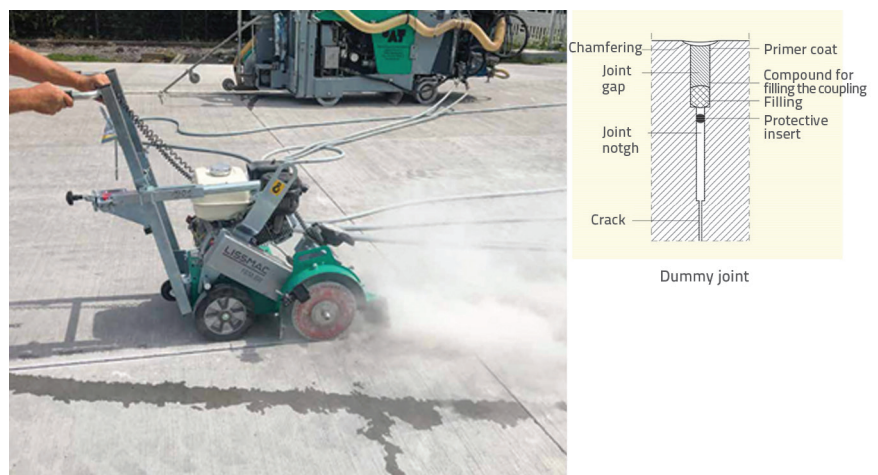
Figure 14. Joint cut: Haunch milling (chamfering) in the foreground. In the background, the ride-on cutting machine for the previously created first and second joint cut (1 st joint notch, 2 nd joint gap) [3]
