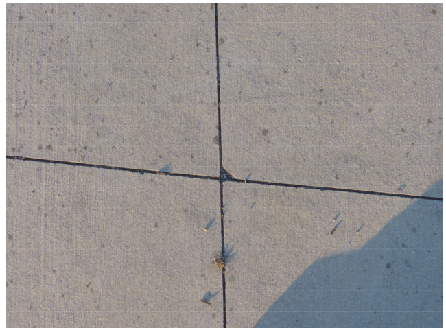
Figure 2. A concrete road surface showing no ruts with significant water accumulation [author, 2016]
