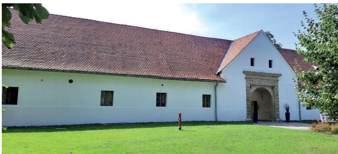
Fig. 8 Comparative photograph taken before the façade was restored, showing the bare structure of the building - the brick construction of the manor house, and later, when the façade has been completed and protects the construction of the building (photography by Tajda Benko).
