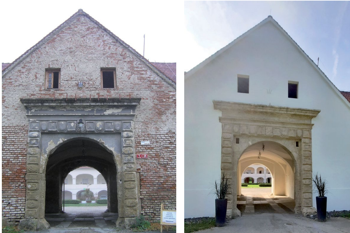
Fig. 5 The portal in the context of the entire eastern wing (formerly utility wing) before and after the restoration of the façade and portal (photographs by Tajda Benko and Andreja Benko).
