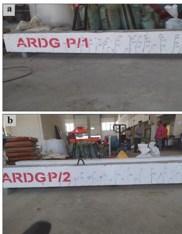
Figure 6 Flexural and shear cracks of parabolic post-tensioned beam (a) POSTTENP/1, (b) POSTTENP/2
