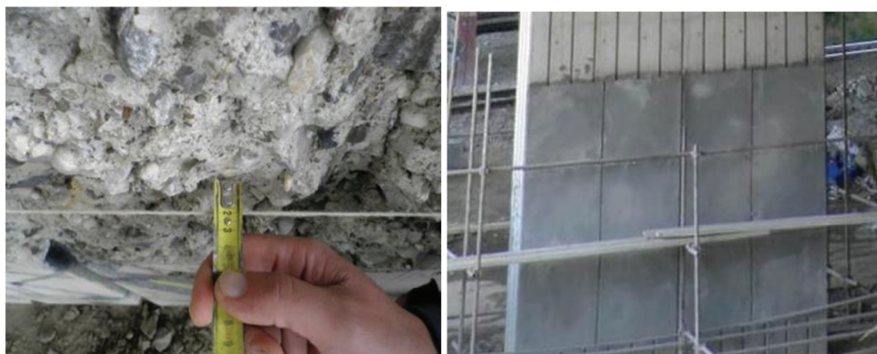
Fig. 4: Appearance of concrete surface after surface preparation by hydrodemolition under high pressure (left) and test fields before pull off testing (right).
