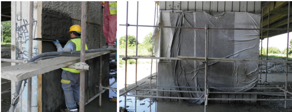
Fig. 3: Finishing of repair mortar surface (left) and curing of repair mortar (right).
