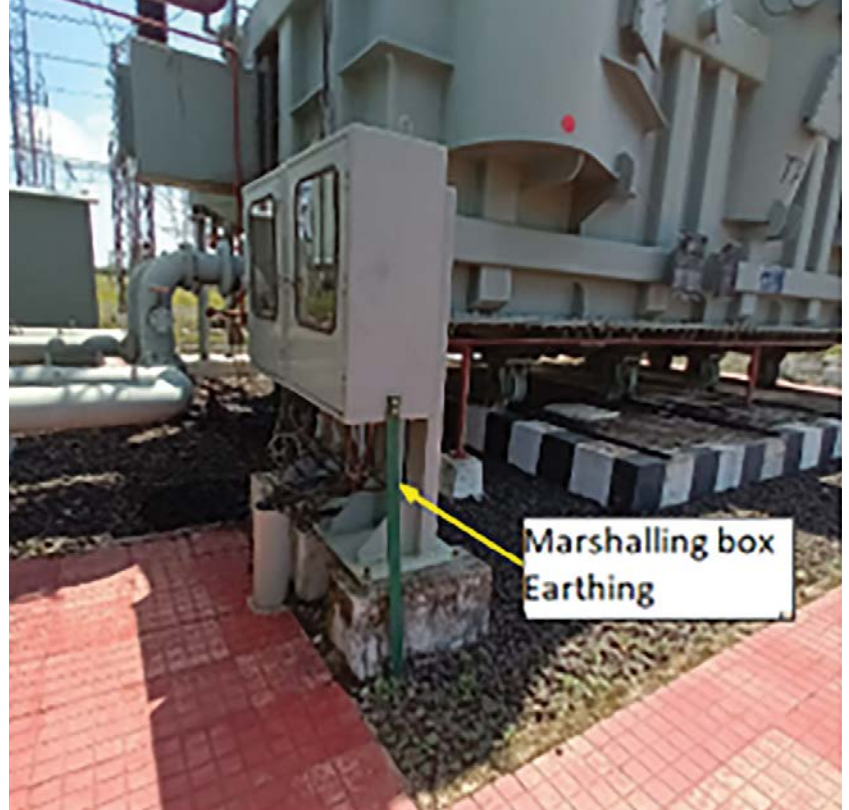
Figure 16D. Marshalling box earthing
