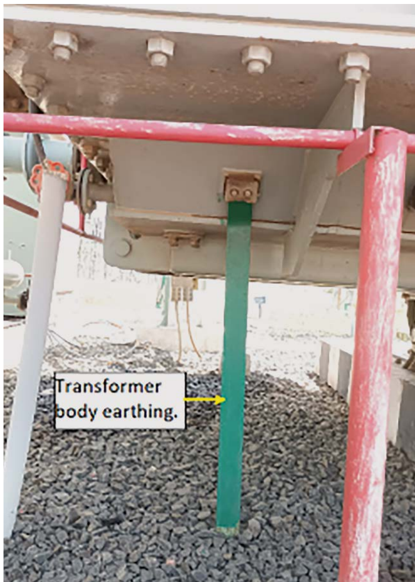
Figure 16C. Transformer body earthing
