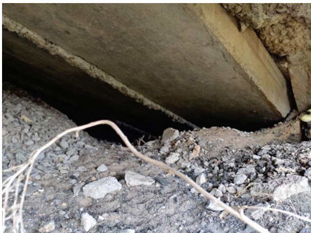
Figure 2 Soil spillage under the approach slabs in the area where the bridge meets the approaches due to precipitation - View from the road side
