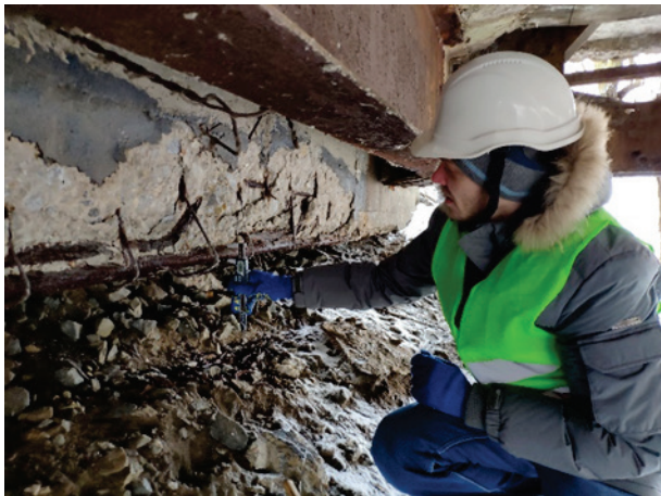
Figure 1 Soil spillage under the approach slabs in the area where the bridge meets the approaches due to precipitation - View from the side of the bridge pillar
