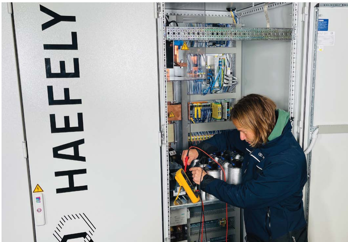
Proactive Maintenance for HAEFELY Systems
