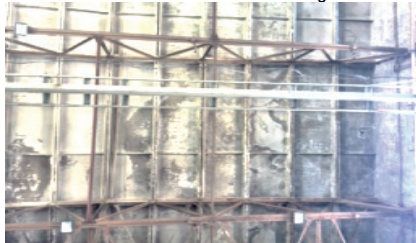
Roof flowing with intensive corrosion damages of trusses elements
