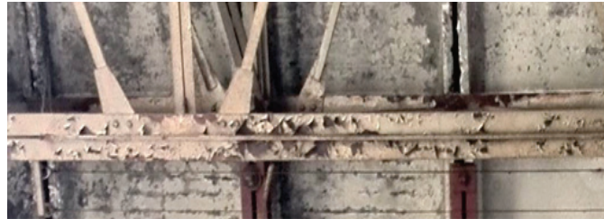
25-30% corrosion of trusses elements cross-section
