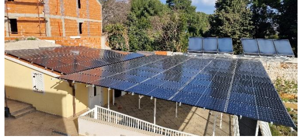
FIGURE 1: EXISTING PV SYSTEM SOLAR-1
