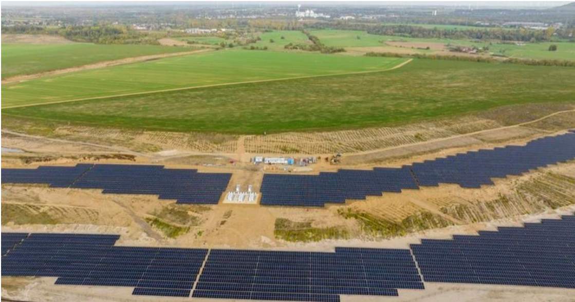
Figure 4. RWE Indeland solar plant Inden, Germany [30]
