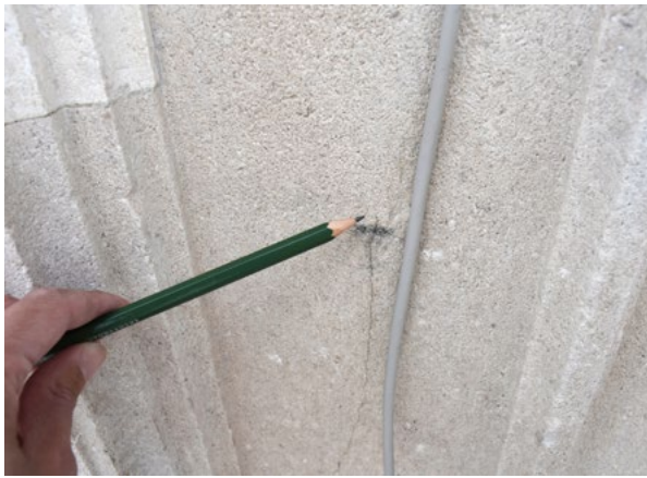
10. Orlando's Column, pillar, east side, vertical crack in 2021 (HRZ Archive, V. Marinković, 2021)
