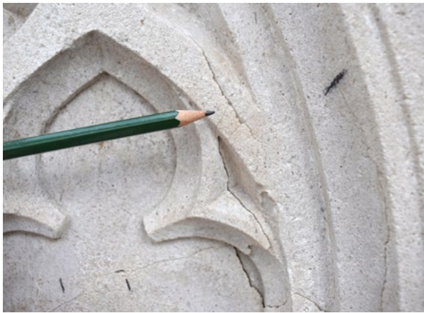
11. Orlando's Column, pillar, east side, unstable damage in 2021 (HRZ Archive, V. Marinković, 2021)
