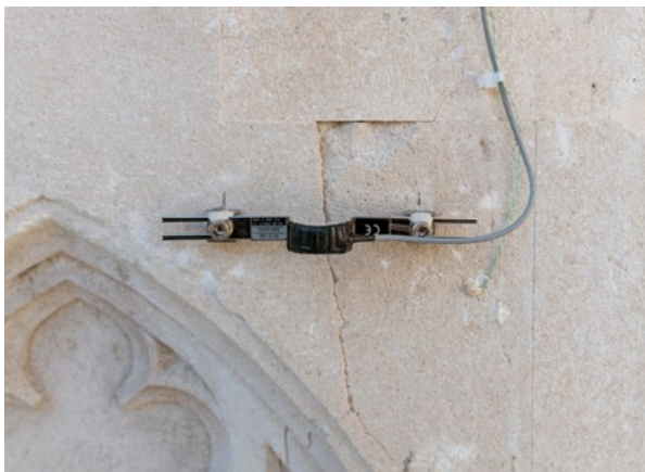
12. Orlando's Column, pillar, east side, sensor for measuring the displacement of cracks (HRZ Archive, P. Gamulin, 2021)
