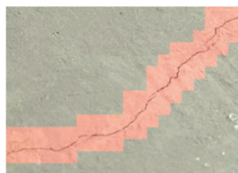
Figure 8 Schematic of concrete crack detection results
