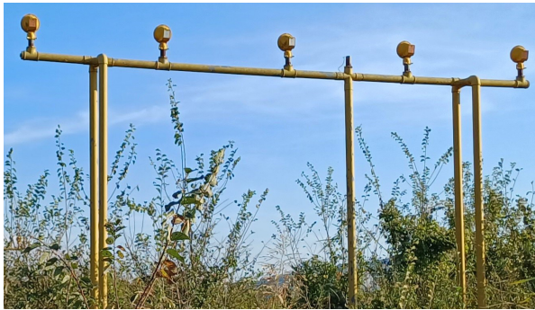
Figure 8 Pillar type „II“ with pipe-structure and crossbar for the approach lights of Tivat Airport, [13]
