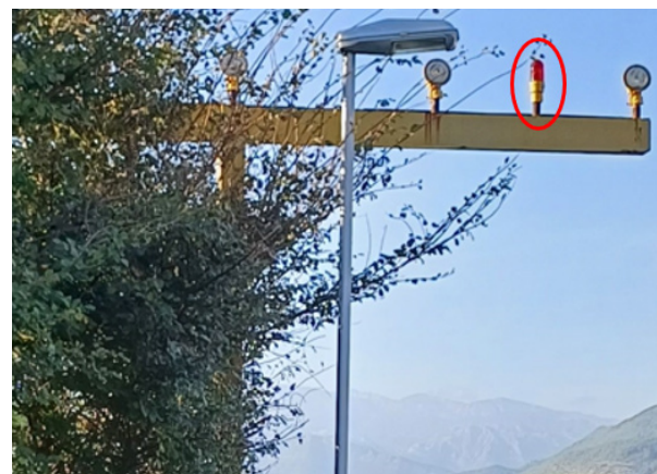
Figure 7 Pillar type "T" with approach lights and a single light for obstacle marking Tivat Airport, [13]
