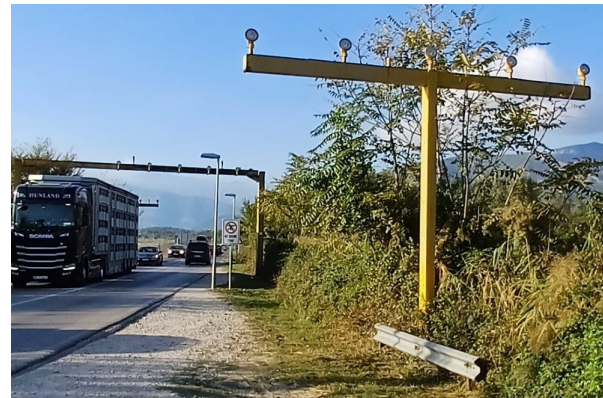
Figure 5 "T" pillar with five lights on the approach lighting crossbar Tivat Airport alongside the road, [13]
