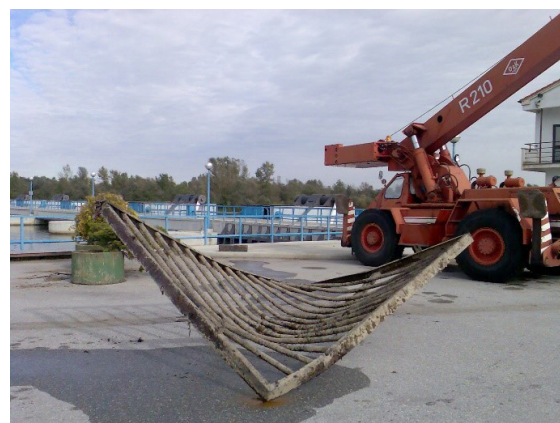
Slika 8. Deformirana gruba rešetka agC HE Varaždin Figure 8. Deformed rough grid agC HPP Varaždin
