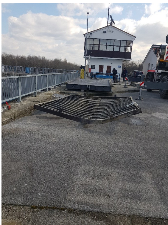
Slika 10. Deformirana nova gruba rešetka agC HE Varaždin Figure 10. Deformed new rough grid agC HPP Varaždin
