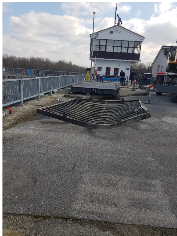
Slika 16. Novoizrađena rekonstruirana gruba rešetka agC HE Varaždin Figure 16. Newly constructed and reconstructed rough grid of agC HPP Varaždin
