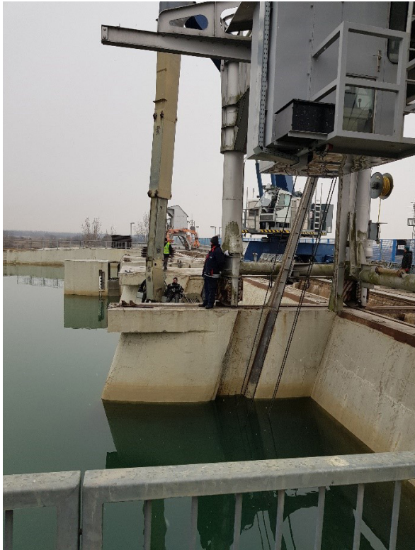
Slika 1. HMO oprema HE Varaždin - dvije čistilice i dizalica za postavljanje zapornica Figure 1. HMO equipment of HPP Varaždin - two cleaners and a crane for installing the shutters
