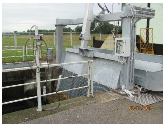
Slika 20. Čistilica MHE Čakovec Figure 20 MHP Čakovec treatment plant
