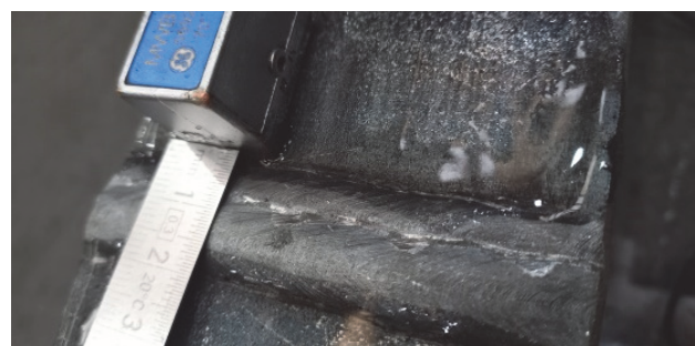
Figure 13 Measuring defect location on the examined weld no. 1
