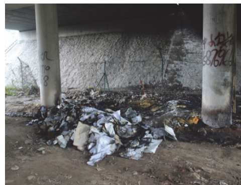
Figure 8 Post disaster condition under the bridge
