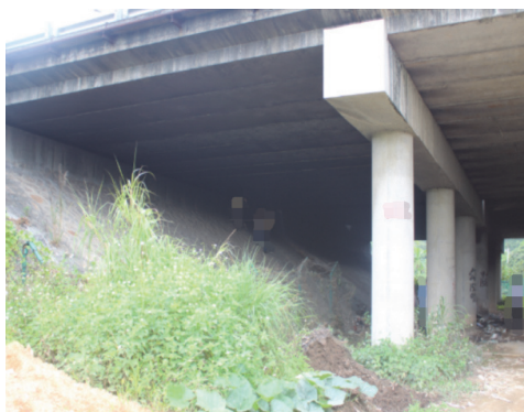
Figure 4 Bridge bottom illumination
