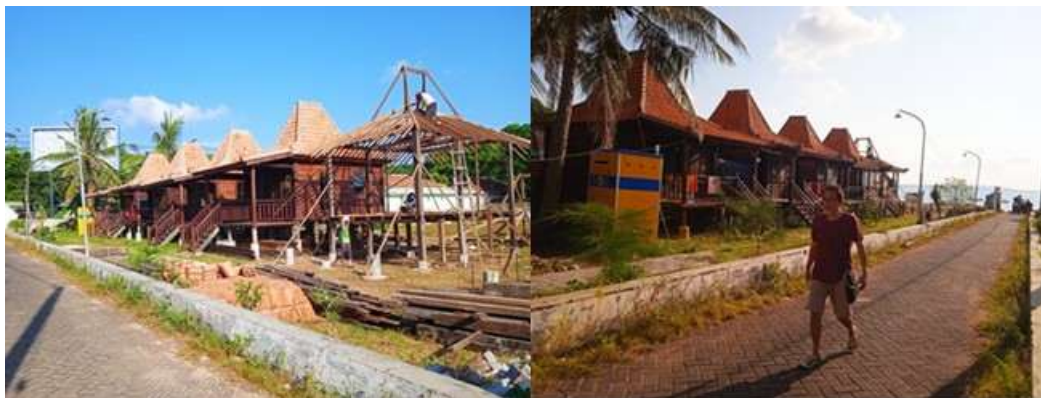
Figure 11. Homestay built near Banra'as Pier for visitors to stay on Gili Iyang Island under construction (Source: personal document)
