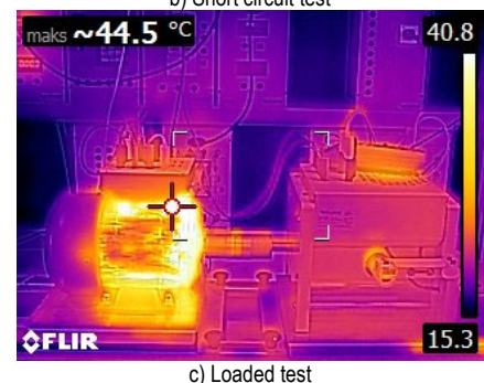
Figure 5 Thermal images of the faulty motor
