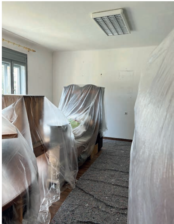
Figure 6. The central room of “Bakina hiža” after completing the works (photo by the author, July 2024)
