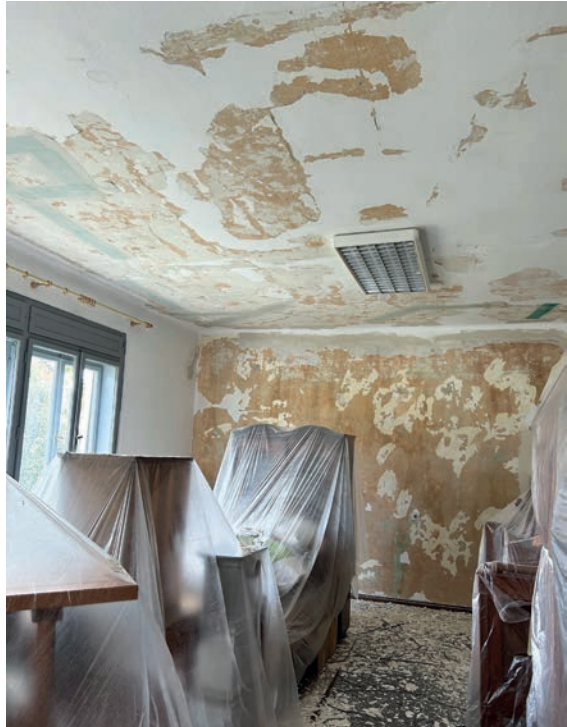
Figure 5. The central room of “Bakina hiža” before the works (photo by the author, June 2024)
