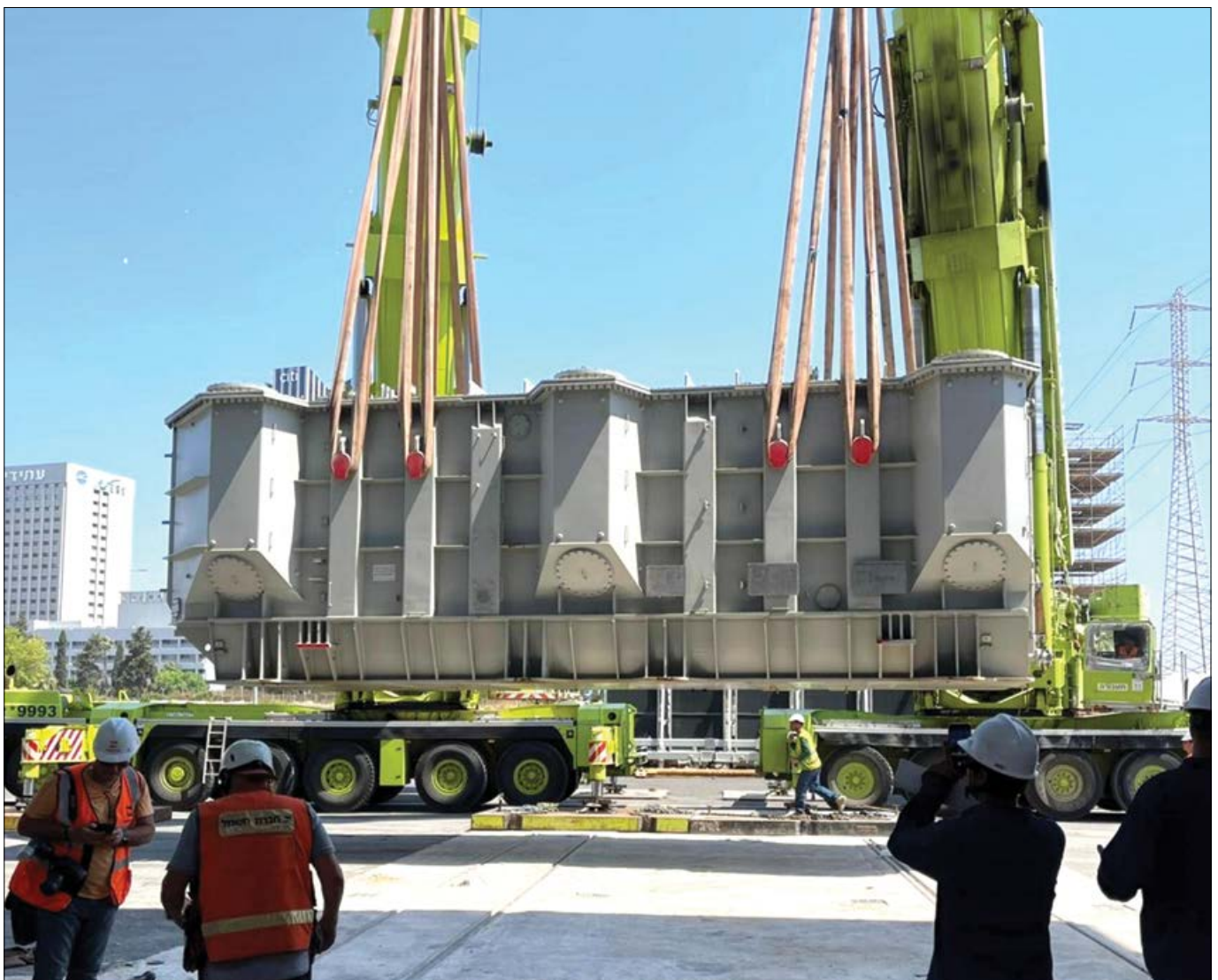
Figure 2b. Transportation of a high-power transformer
