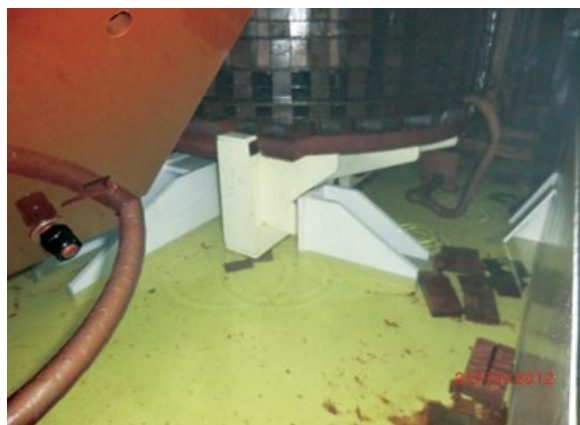
Figure 7. Active part displacement of 63 MVA, 220/110 kV autotransformers cover
