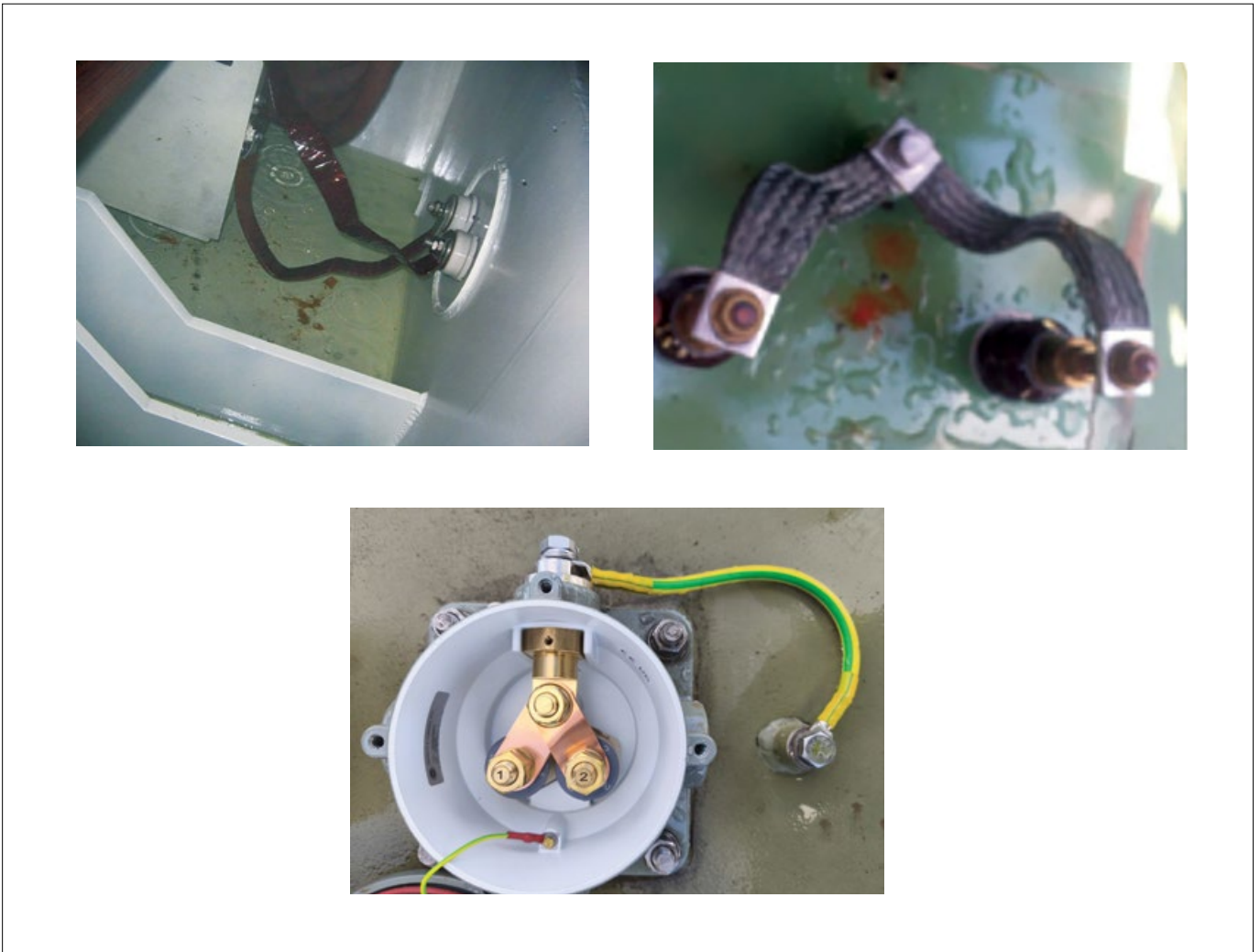
Figure 3. Grounding output unit core and frame (view from inside the tank and on the tank cover)
