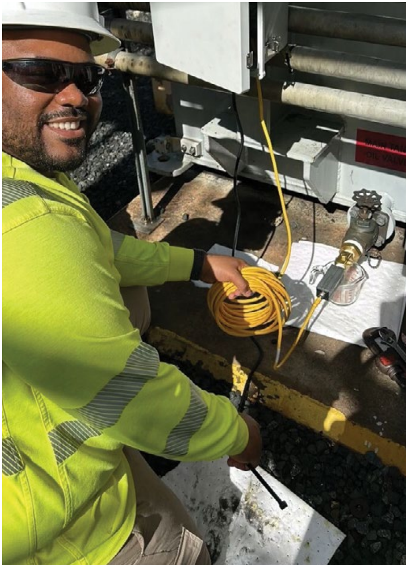
Figure 2. Installation of the continuous monitoring sensor took fewer than two hours to complete without requiring an outage or power shutdown.
