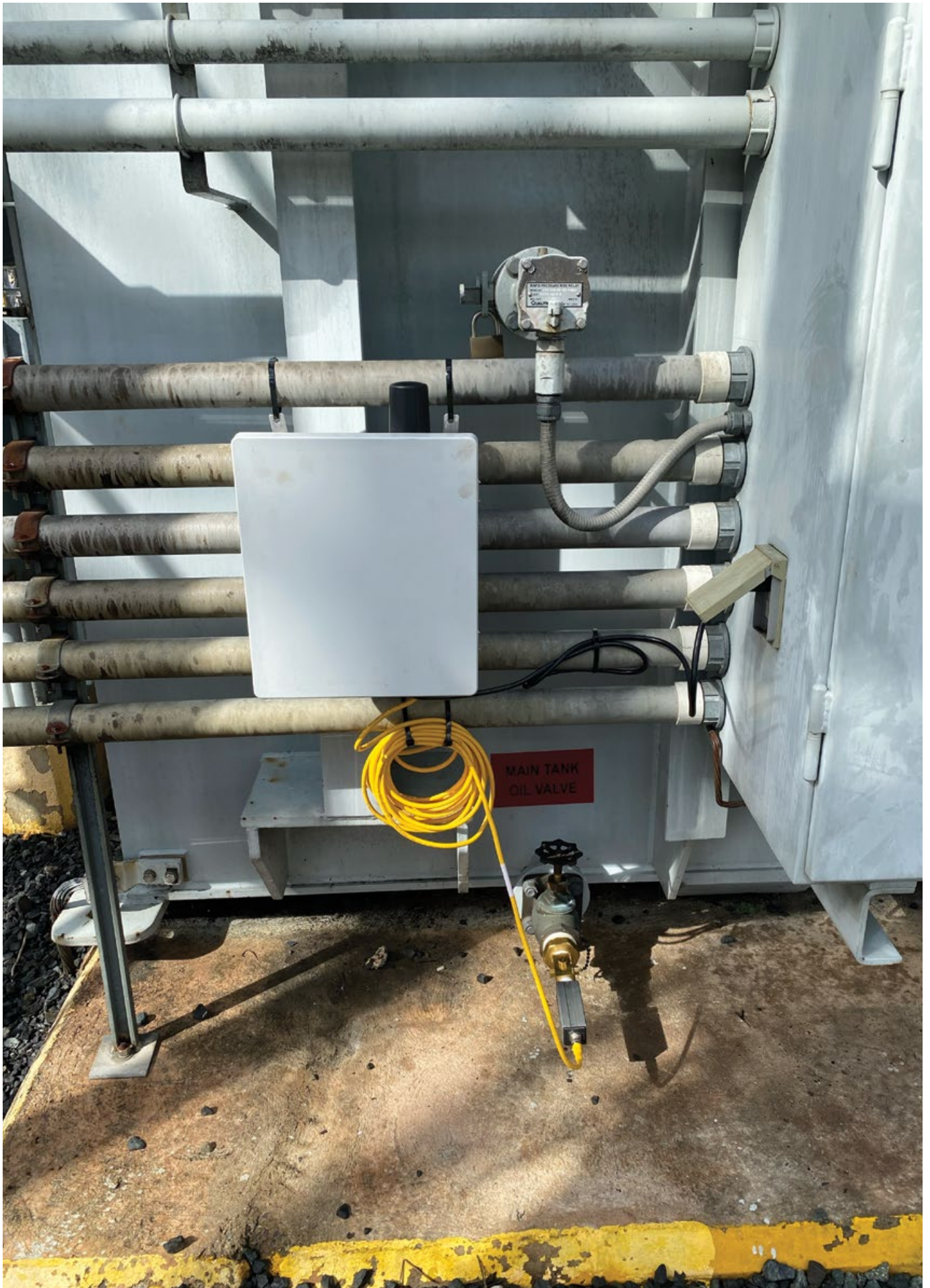
Figure 3. Final installation of the H2scan GRIDSCAN® 5000 hydrogen sensor, which requires no periodic calibration. Workers should not have to return to the sensor for at least ten years, minimum.
