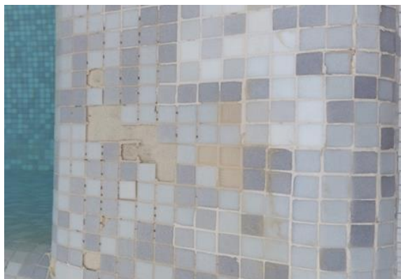
Figure 2. Appearance of damaged pool tiles caused by cleaning with technical HCl (10 w/w%)
