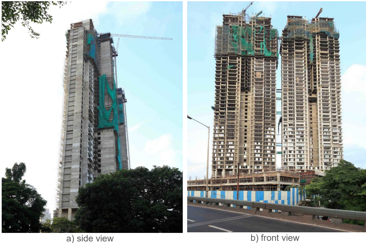
Figure 2. Actual view images for selected case study: a residential tower
