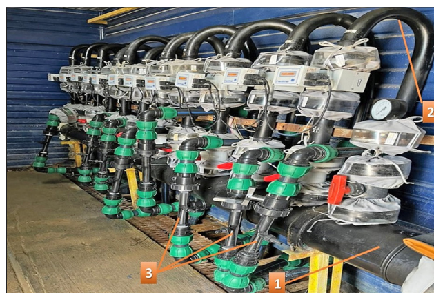
Figure 2. Specialized injectors installed on the lixiviant line via a bypass connection: 1 – main pipeline; 2 – injection well pipeline; 3 – specialized injectors.
