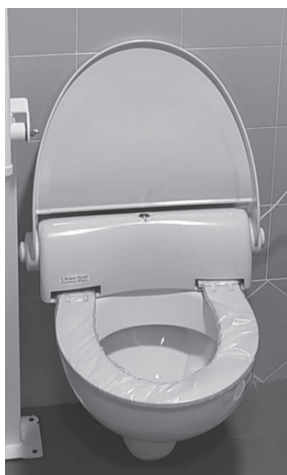
Figure 1. The NAVISANI automated toilet seats were installed inside the administration units
